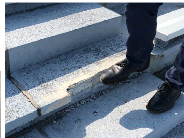
F – Bleacher deterioration
