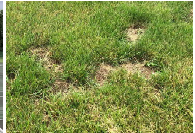
C – Football turf trip hazards
