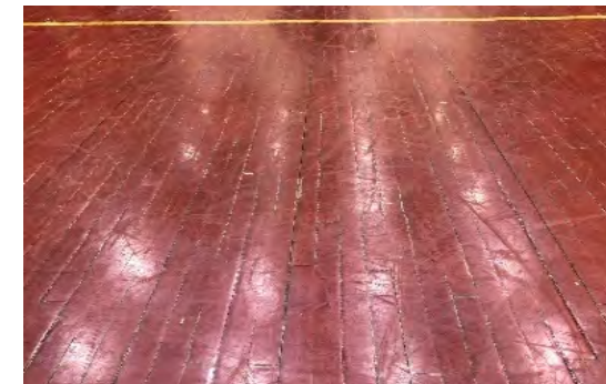
D – Gym floor wear
