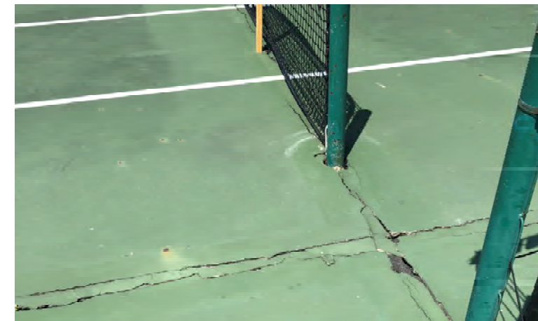
D – Tennis Court cracks
