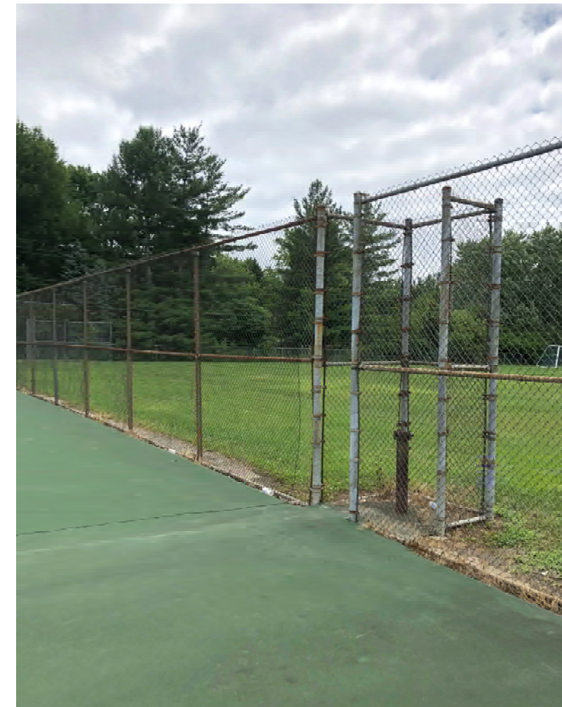
C – Tennis Court & fencing worn
