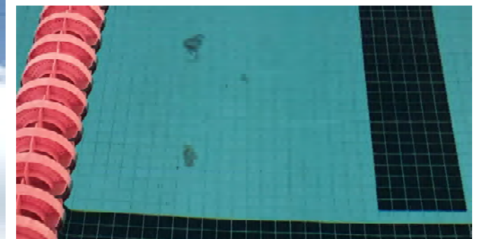
D – Broken tile in tank
