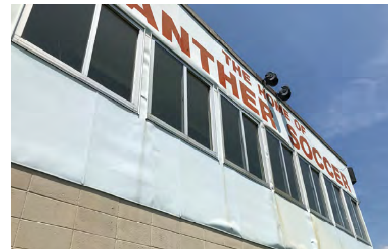
D – Soccer Press box water damage
