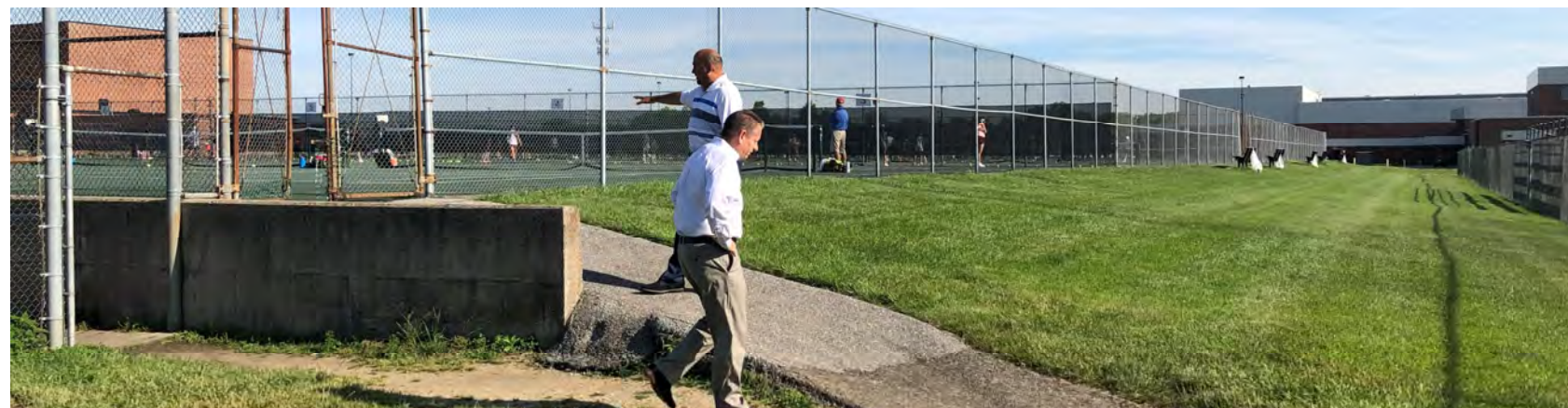
F- Elevation changes and poor drainage
