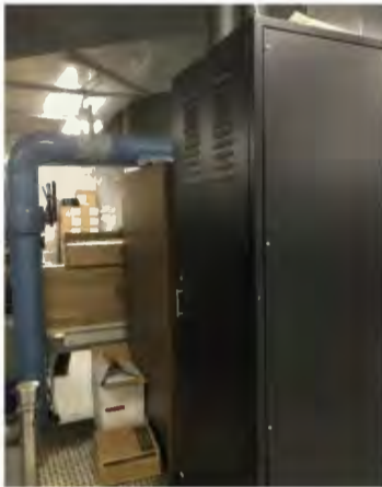
IDF-6 located in large mechanical room on the second floor.
