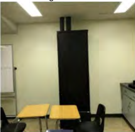
IDF-3 located in “storage room” converted into a classroom in unit G.
