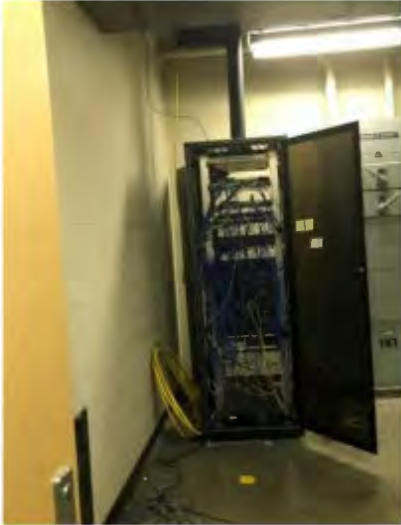
IDF-2 located in an electrical room within classroom in unit G
