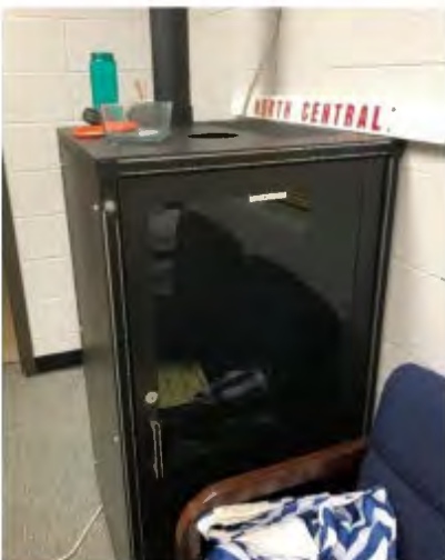
IDF-4 located in gym teachers office off of auxiliary gymnasium.
