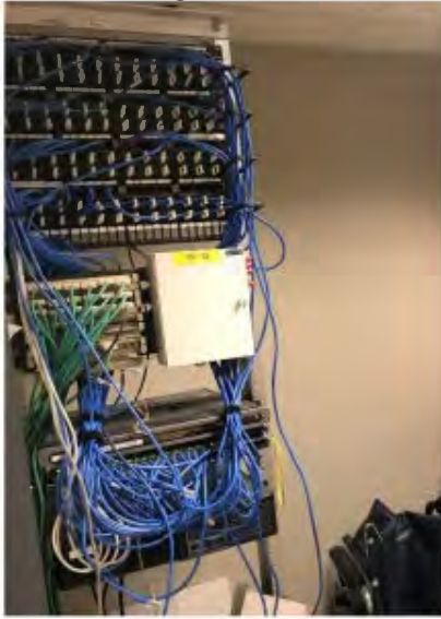
IDF 2 – Storage Room A105C
