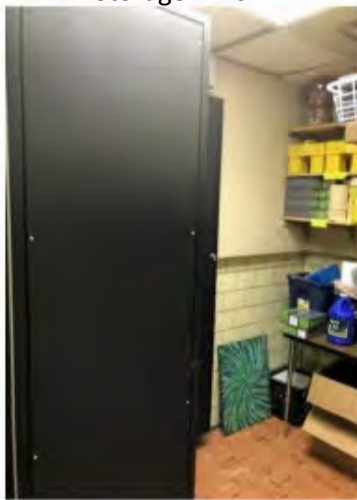
IDF-7 located in storage room on second level. Room used for general storage.
