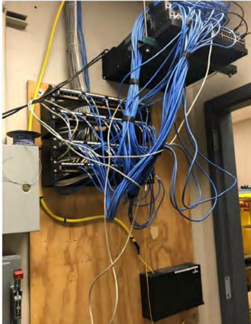
IDF 12 – Electrical Room B119A
