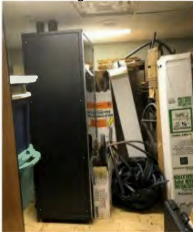
IDF-5 located in storage room on second level of the building. Room used for general storage.
